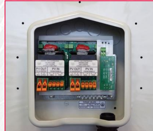
Rapid Shutdown (Micro-inverters) & DC Optimisers
